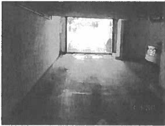
Water marks/stains at basement slab
