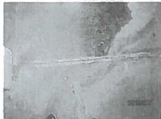
Water marks/stains at basement slab
