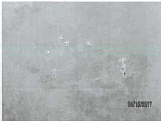
Cracks with water intrusion signs at underside of pool deck
