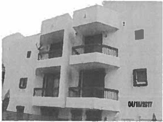
Overflow scuppers without downspout
