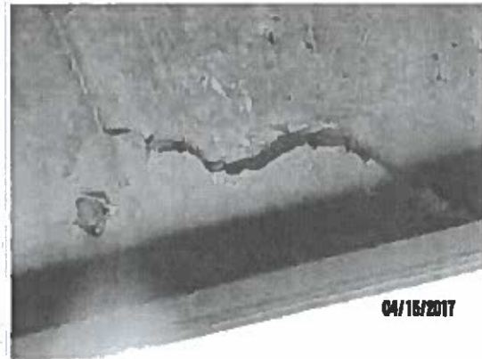
Spalled concrete at underside of pool deck
