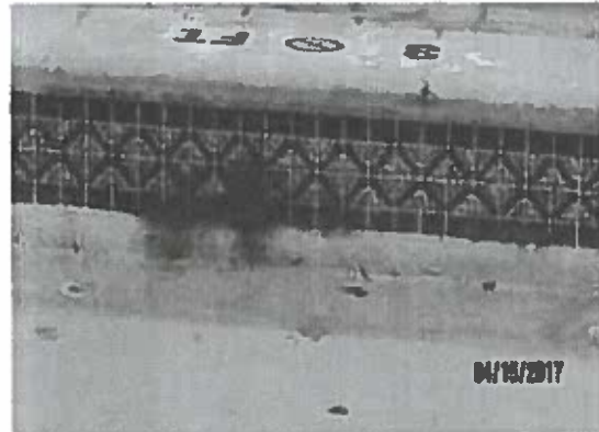
Corrosion at North wall of pool
