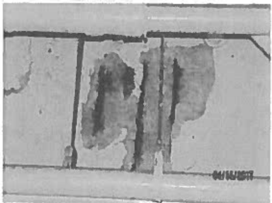
Damaged pool wall at Basement
