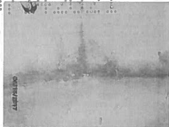
Water marks/stains at basement slab
