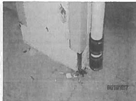
Exposed and corroded column steel reinforcement
