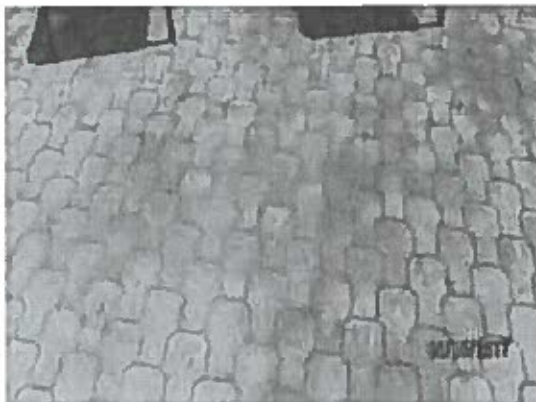
Water/stain marks at pool deck pavers
