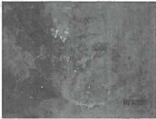
Cracks with water intrusion signs at underside of pool deck
