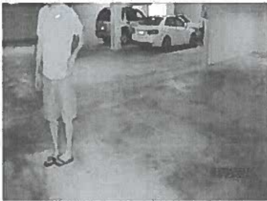
Water marks/stains at basement slab
