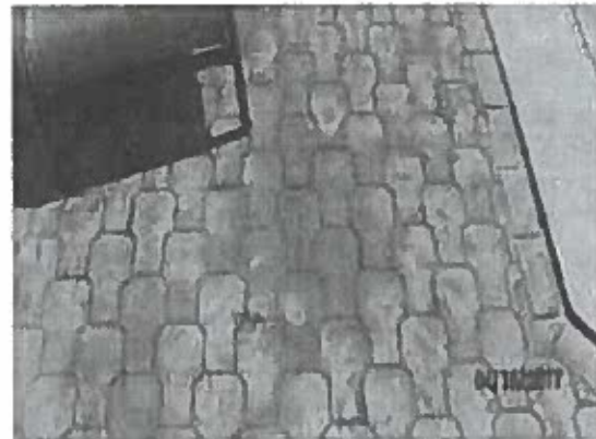
Water/stain marks at pool deck pavers
