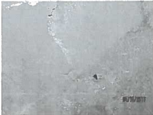
Spalled concrete at underside of pool deck
