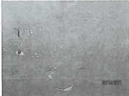
Spalled concrete at underside of pool deck
