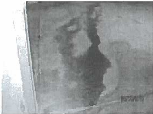
Water marks/stains at basement slab
