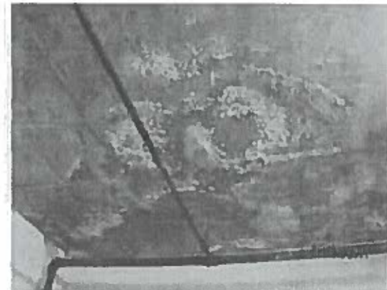
Water intrusion signs at underside of pool deck
